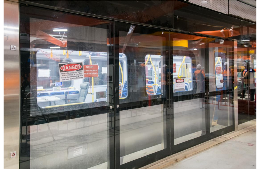
Victorian-first platform screen doors have been installed at each Metro Tunnel station for better safety, climate and noise control.
